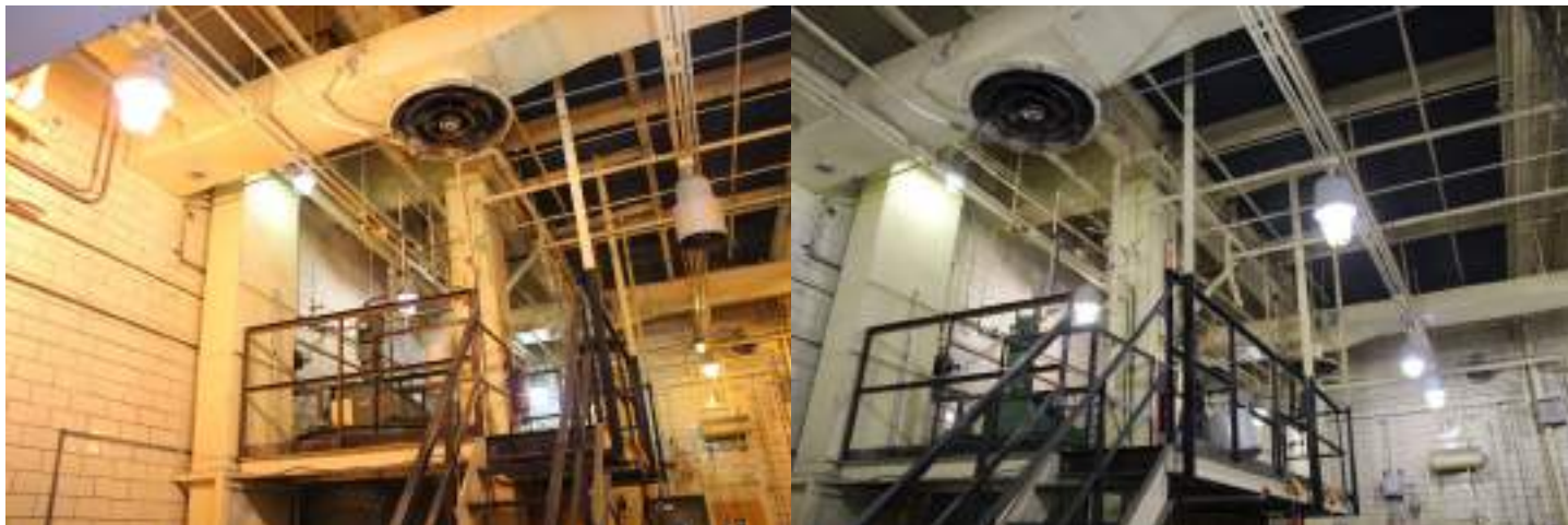
Before: 250W High Pressure Sodium Lamps
